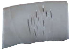
Hose with cover cracks due to age or the effects of ozone. Hose covers over time harden and should be replaced if this condition is found. (note: if boat has an ozone generator on board this could accelerate this condition
