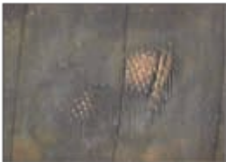
Exhaust hose with cover worn, exposing reinforcement
